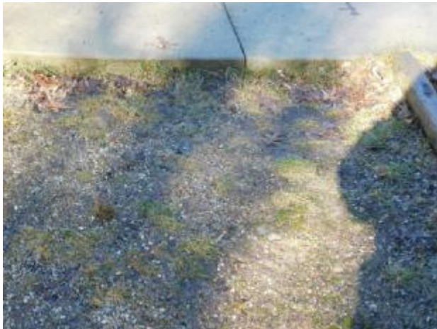
Uneven ground at driveway
