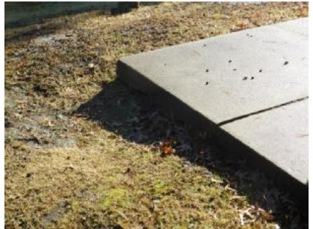
Uneven ground front walkway
