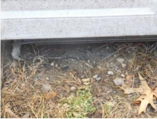
Gap at garage door
