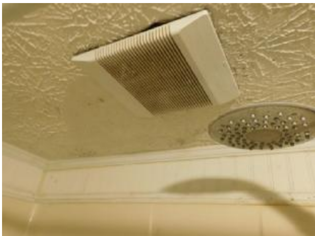
Non-working exhaust vent
