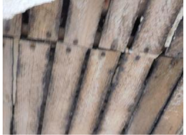
Falling ceiling in back bedroom
