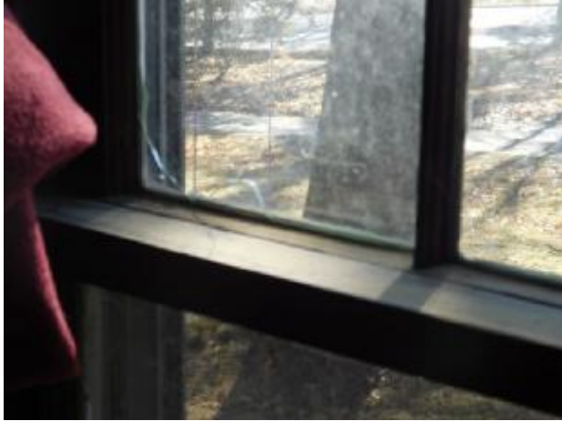
Cracked glass in dining room
