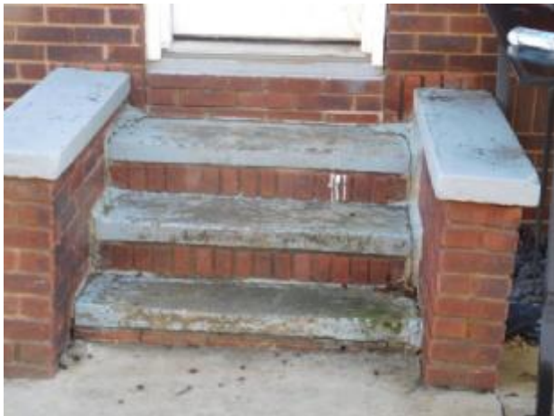
No handrail at back entrance
