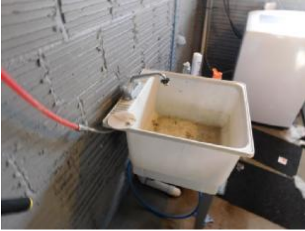
Not mounted/ improper supply line
