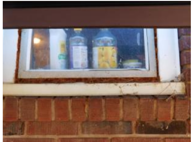
Window does not operate/foam
