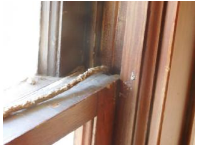
Broken sash cord back bedroom
