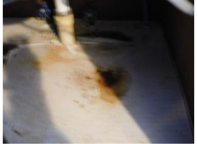
Signs of previous leak
