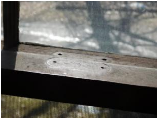
Missing lock back bedroom window
