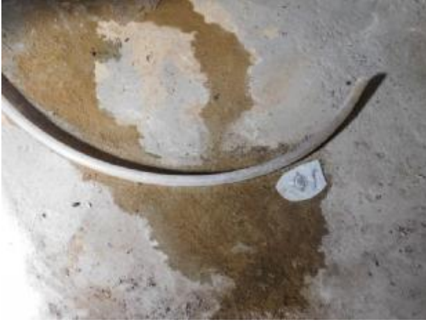
Improper AC drainage
