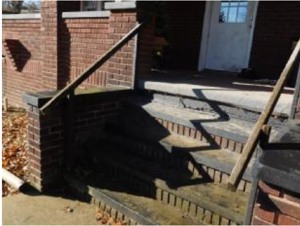
No Handrail at front entrance
