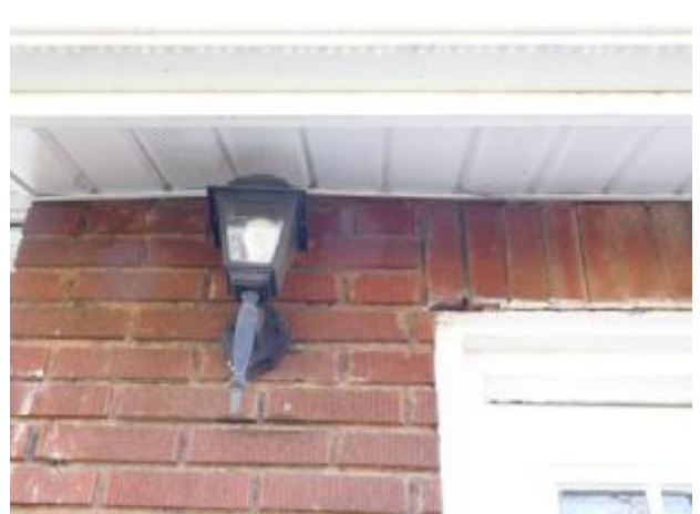
Light not working/missing caulking
