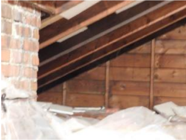
No bathroom vent connection
