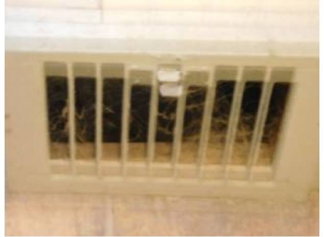
Non-working bathroom vent
